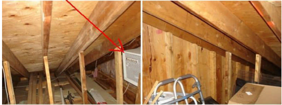
Bedroom Air Conditioner
