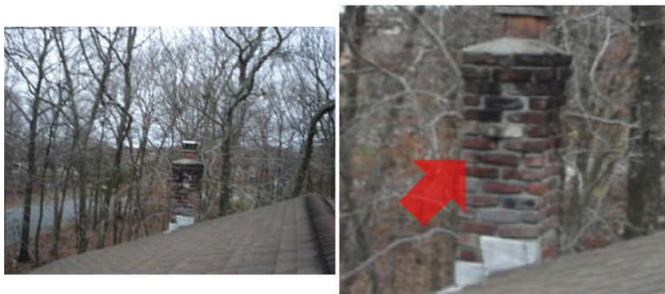
Deteriorating Mortar Joints Brick.
