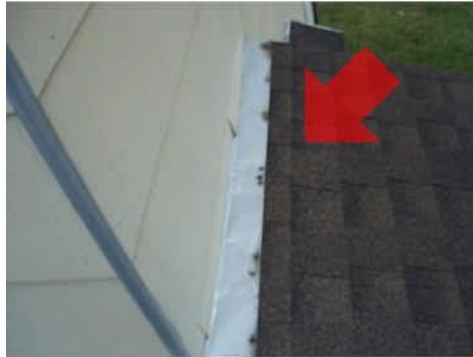
Exposed Nail Heads Metal.
