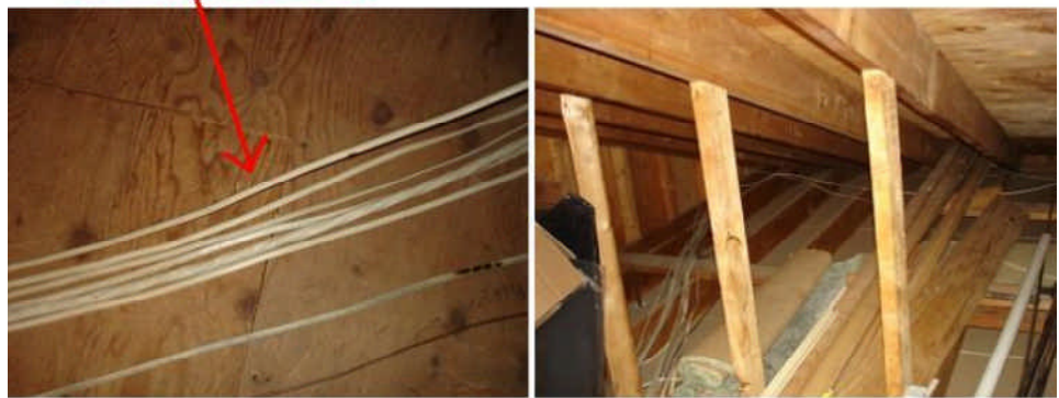
Cabeling On Attic Floor
