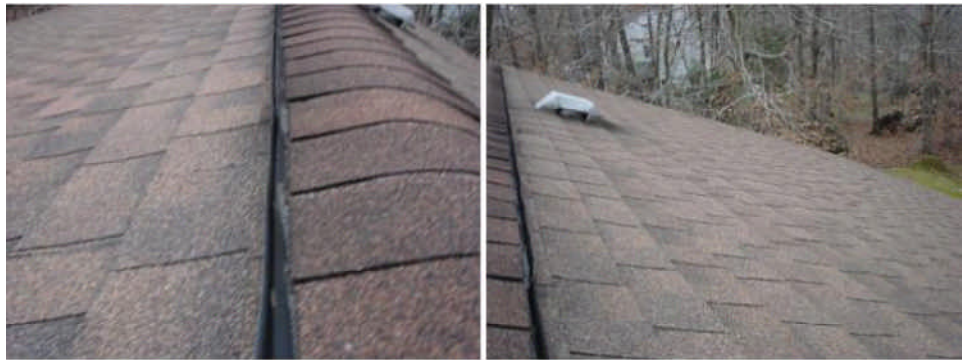
Exposed Nail Heads Composition shingles.
