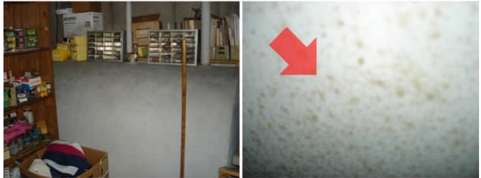
Oil Tank Bottom
